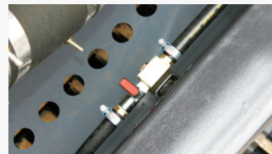
Fuel tank water drainage cock
